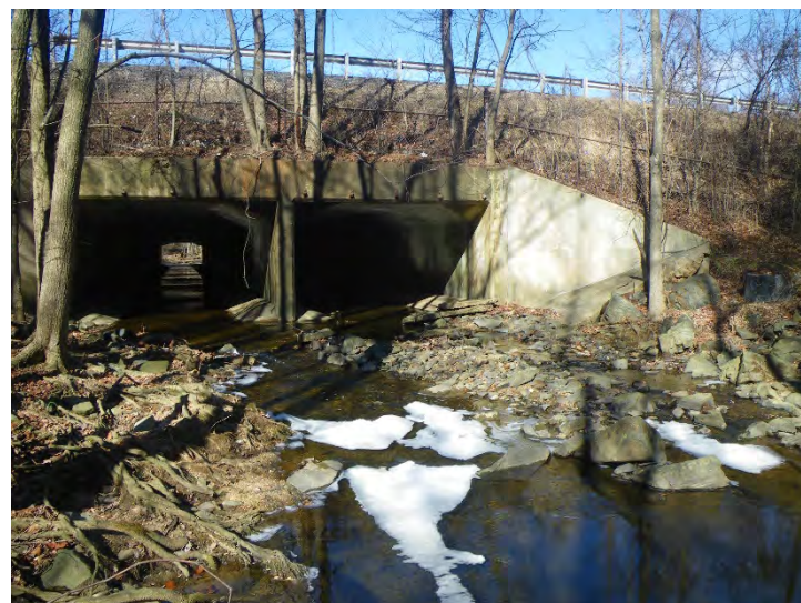
Facing upstream at the downstream face of the I-95 culvert (downstream of I-95), no fish blockages observed.
