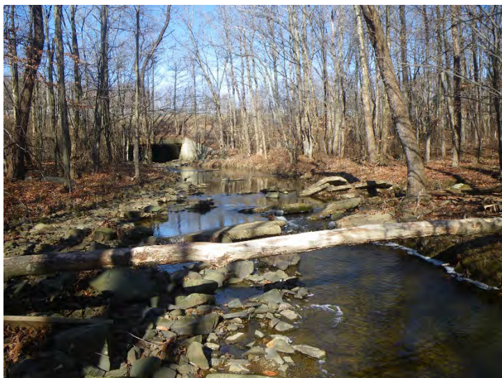
Facing upstream at Carsins Run downstream of I-95 (note broken slabs of concrete).
