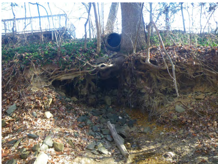
Facing left bank at severe erosion at 21" stormdrain outfall off of Randolph.
