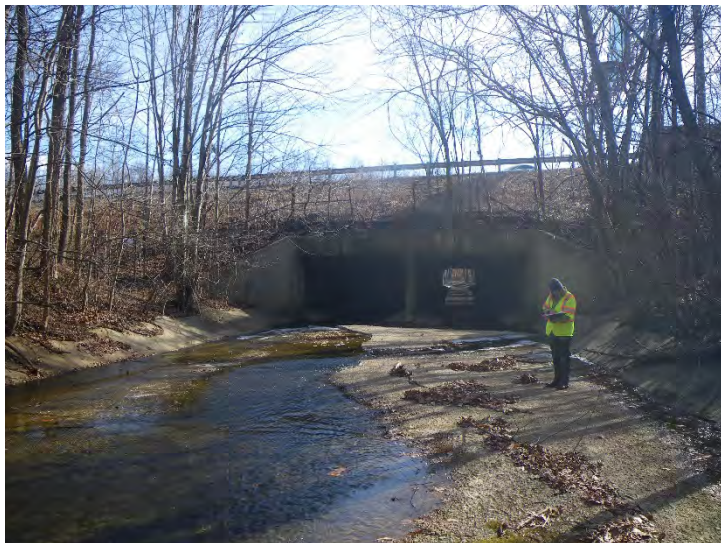
Facing downstream at upstream face of I-95 culvert and concrete lined channel (proposed W-Weir location)
