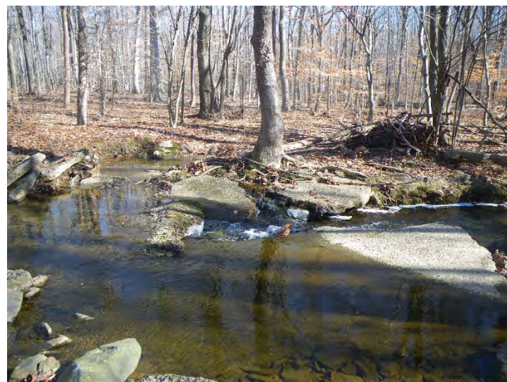
Facing left bank close up of broken concrete slabs.
