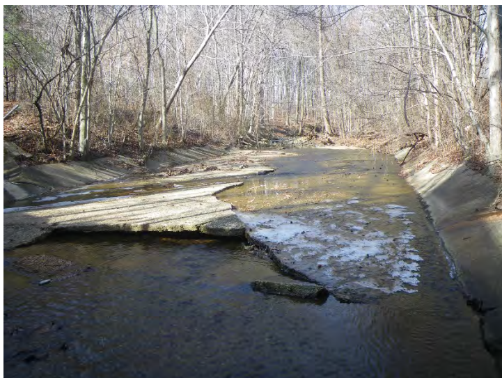
Facing upstream from Sta. 14+44 (invert of upstream end I-95 culvert) showing broken concrete lining to be removed.
