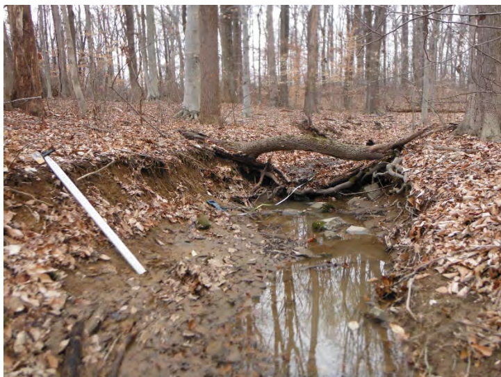
Facing upstream at knick point/headcut. Note, the fines and right bank erosion (~Sta. 7+75).
