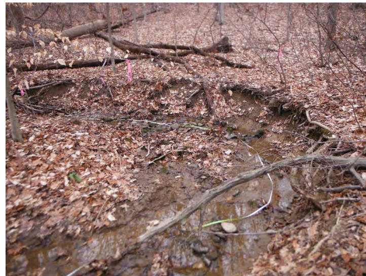
Facing upstream from near 5+50 at typical bank erosion.
