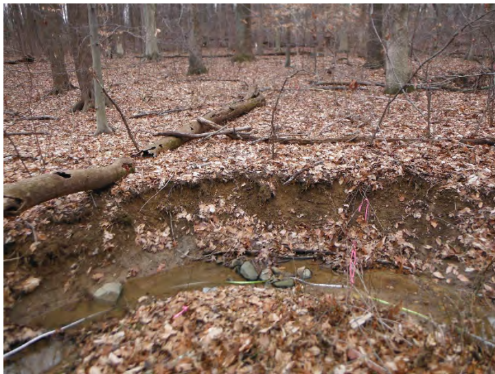
Facing right bank at typical outer bend bank erosion in Reach 3 (from Sta. 6+30)
