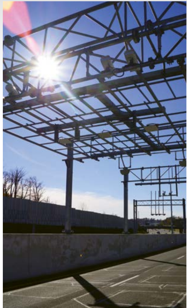
I-95 ETL TOLLING GANTRIES
