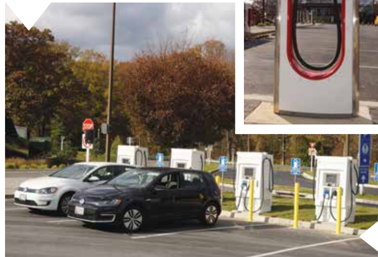
Charging stations at the Maryland House and Chesapeake House travel plazas
