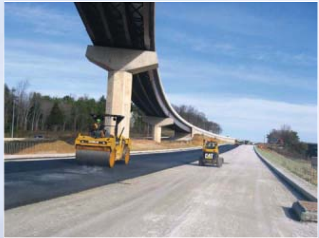
Southbound I-95/I-695 General Purpose Lane construction. The overhead ramp from southbound I-95 to eastbound I-695 opened in June 2009.
