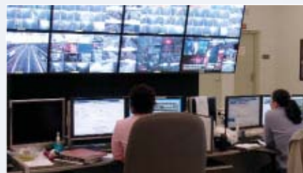
New Central Region Authority Operations Center.
