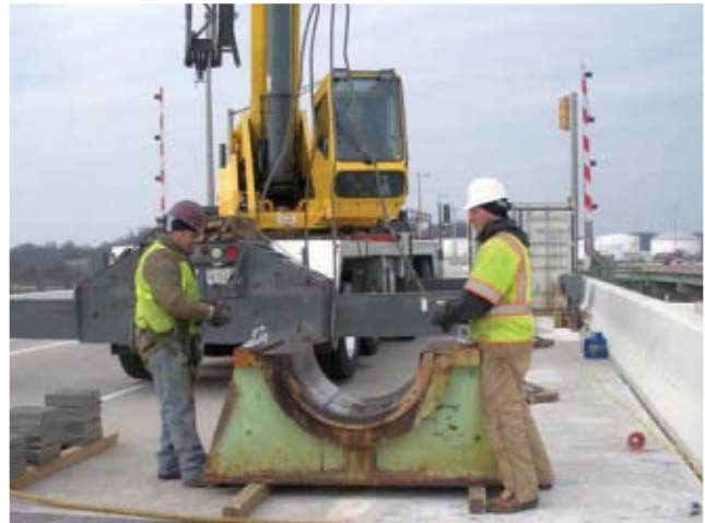
Trunnion bearing is removed in preparation for Curtis Creek drawbridge repair, near the Key Bridge.
